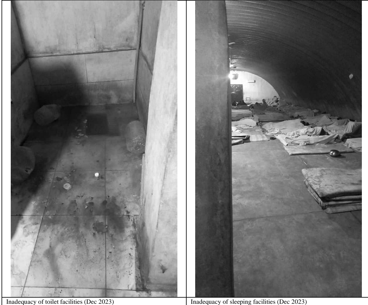
Inadequacy of toilet facilities (Dec 2023)
