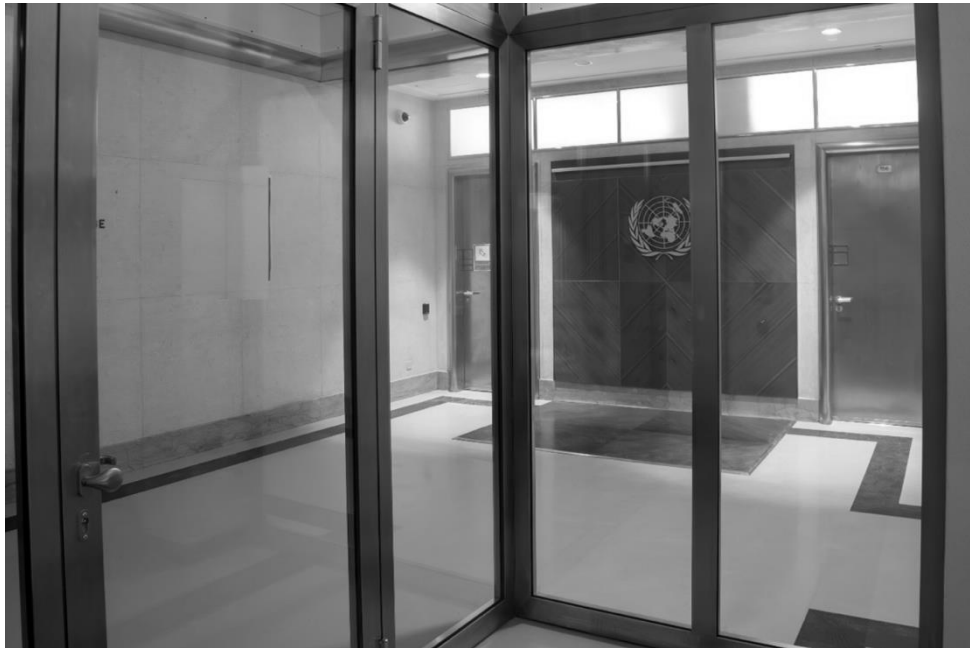
Figure VI Interior showing newly created fire and smoke compartmentalization in the renovation of heritage building S, April 2024
