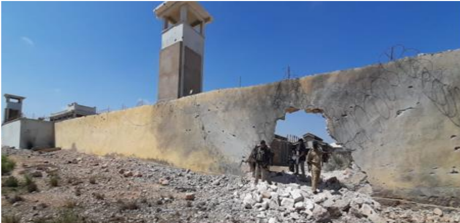
Figure 2: Hole blasted into the eastern prison wall.
