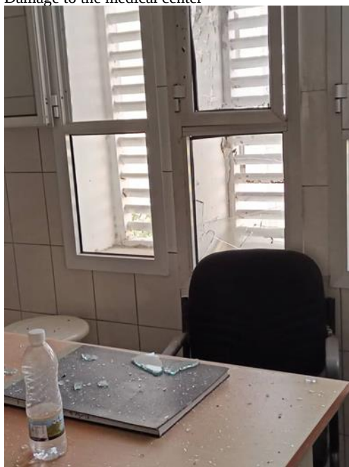
Figure 33.4: Damage to the medical center
