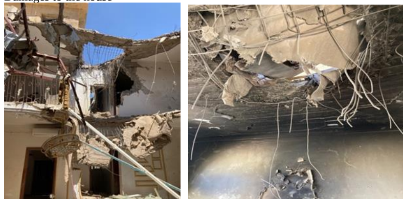
Figure 33.6: Damages to the house
